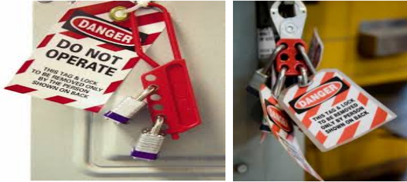
Figure 3: Example of multiple locks on a lockout tag.
